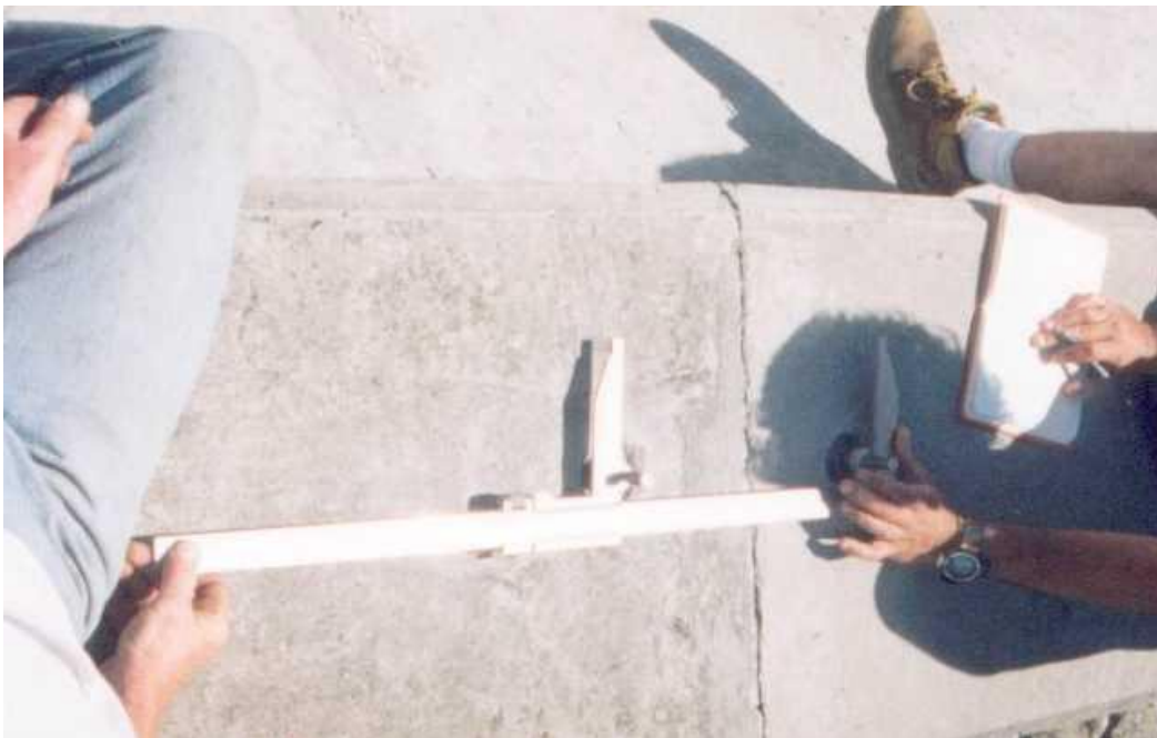
Figure 7-5. Starrett vernier caliper crack measurements between monoliths. Central & Southern Florida Flood Control Project (Jacksonville District and Arc Surveying & Mapping, Inc).
