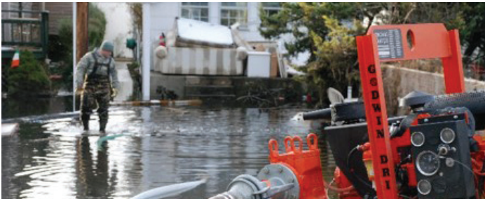
Pumps utilized for dewatering operations in flooded areas caused by Hurricane Sandy.
