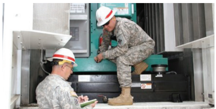
Engineers working on the generators during Hurricane Sandy Disaster Relief Response
