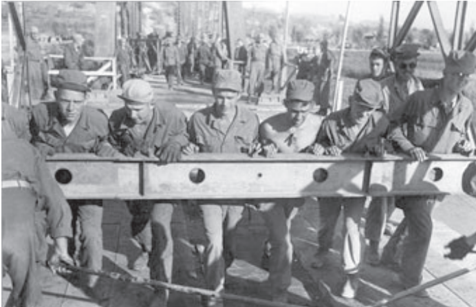
Engineers build a Bailey bridge across the Naktong River at Waegwan, 1 Oct. 1950
