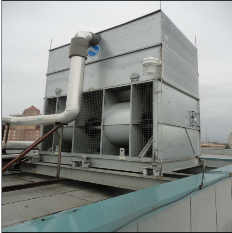
Existing Cooling Tower on Roof of Building
