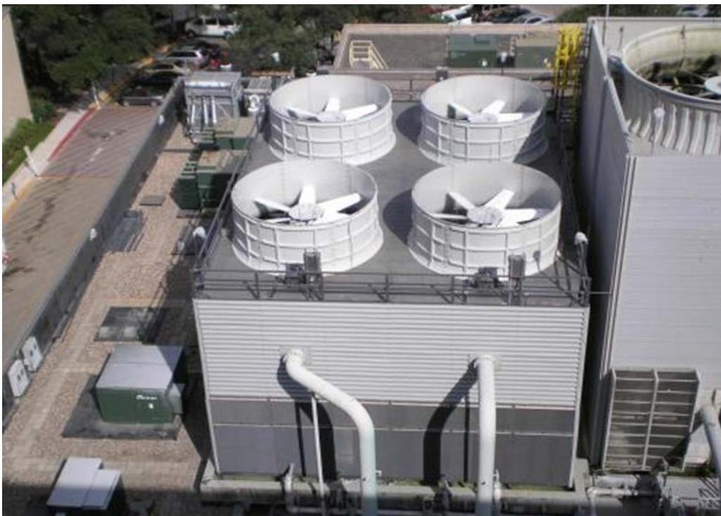
Typical Large Cooling Tower Serving a Hospital
