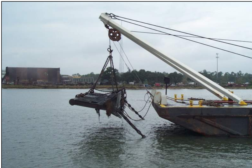
Figure 2-39. Bed-Leveler Suspended by an A-Frame on a Work Barge (Photo Courtesy of Bean Dredging Company, New Orleans, LA)
