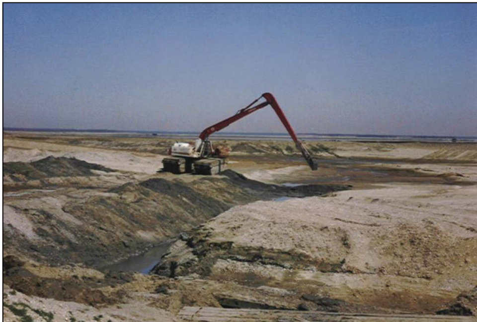
b. Trenching the North Cell of Dredged Material on Hart-Miller Island to Maximize Dewatering, so the Site can be Filled to Capacity prior to Wildlife Habitat Development
