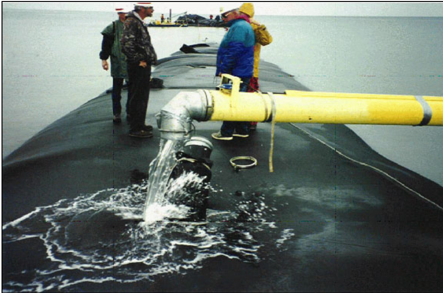
b. Filling a Custom-Designed Geotextile Tube with Dredged Material in Chesapeake Bay, MD, for Erosion Control and Sediment Stabilization
