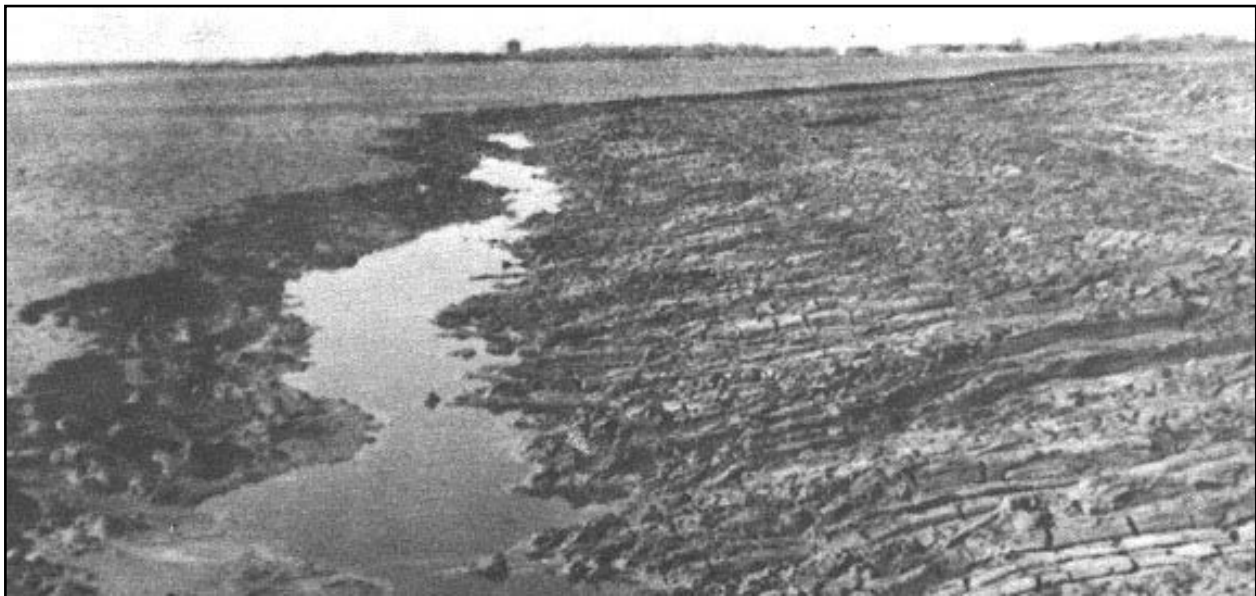
Figure 4-33. Construction of a Ditch 30-45 cm (12 to 18 in.) Deep with Excavated Material Cast on the Interior Slope of a Perimeter Dike
