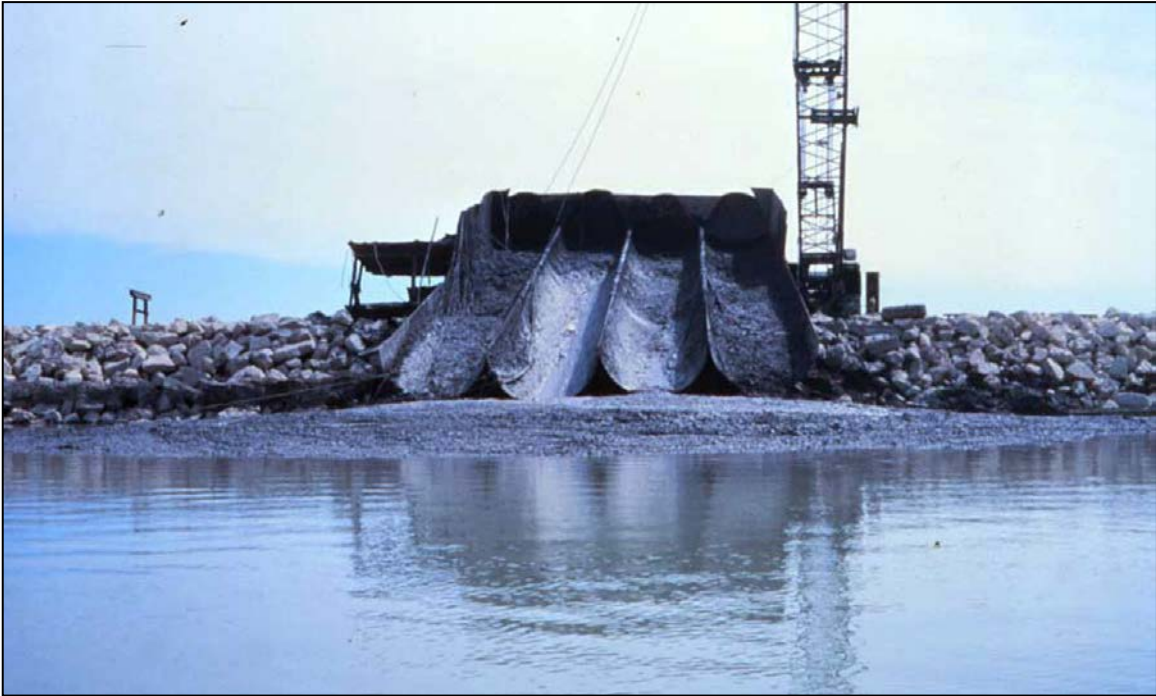
Figure 4-10. Chute Fabricated from Railcar Tanks Used for Direct Mechanical Placement into a CDF
