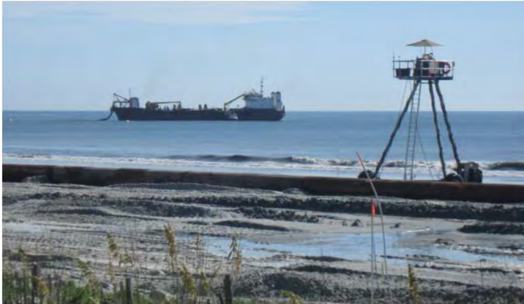
Figure 11-8. One of the CRABs operated by Great Lakes Dredge & Dock on a 2011 Beach Renourishment Project at Jacksonville Beach (Duval County), FL. The dredge in the background is shown at the beach pump-out site. (Jacksonville District).
