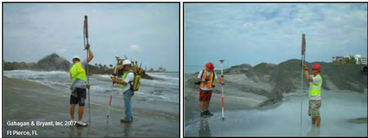
Figure 11-14. Setting a metal grade stake with driving hammer during active beach fill construction. Pre-drilling the stake hole with a portable auger makes for easier driving. RTK stake out observations are used to determine grade levels relative to the template along the profile range. Ft. Pierce Beach Renourishment Project. (Jacksonville District)
