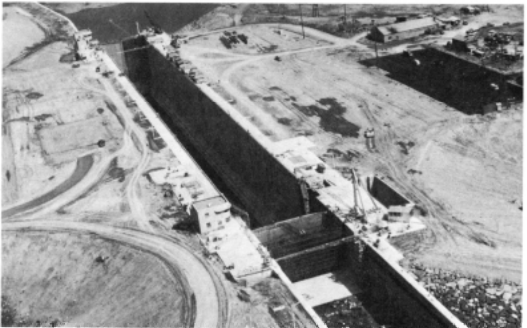
Eisenhower Lock from the north upstream bank, May 1958. Note the upstream miter gate in operable condition and the vertical lift gate in raised position.
