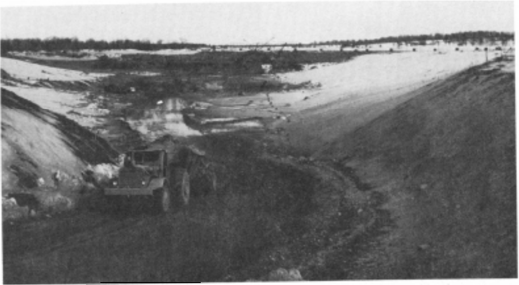
Excavation, from the west end, February 1956. A bottom-dump Euclid in the foreground.
